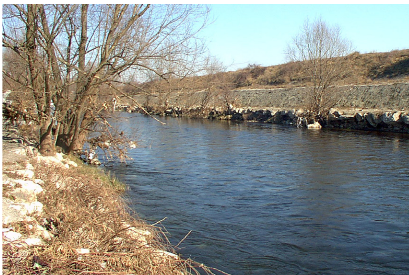
Figure 7 Longitudinal defence in bad status (foot erosion): historical savings on operation, maintenance and replacement imply future harsh problems.
